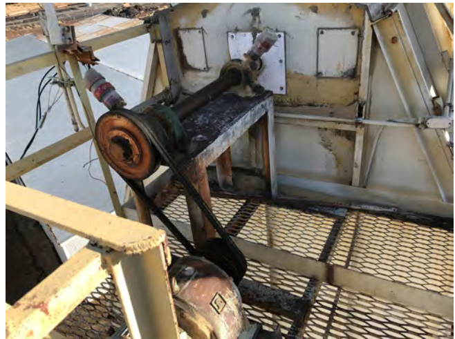
Unguarded incline belt and shaft that powers the sanding machine (shaft rotates at 6,000 rpm).
